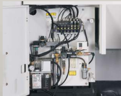
Hydraulic & Lubrication System(LU-620)
